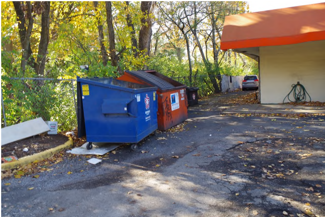
Deteriorated paved surfaces.
