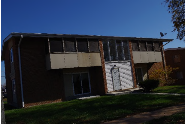
Deteriorated multi-family building.
